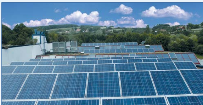
Hevert-Photovoltaikanlage in Nussbaum
